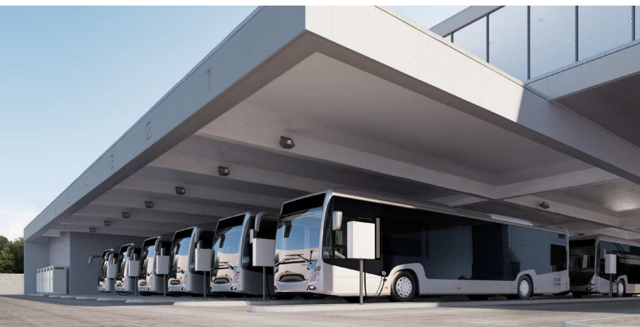
— HVC Depot Boxes and power cabinets, lined up at a depot site.
